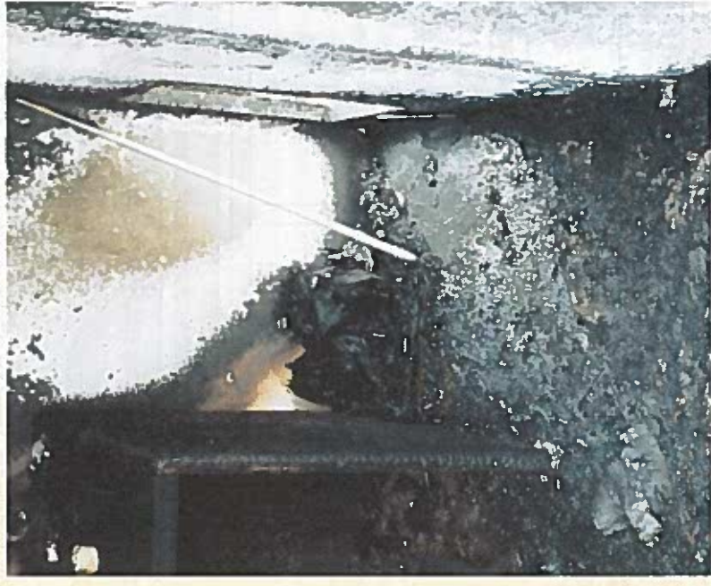
FIGURE 8-9 Results of postflashover fire in a furnished 2.4 m x 2.4 m (8 ft x 8 ft) office cubicle. Note extensive destruction of synthetic carpet and combustion of drywall paper on right. Glass viewport in right-rear corner failed prior to flashover. Note clean-burn ventilation pattern extending up the rear wall, and extensive damage to carpet beneath the opening. There was only carpet and pad in the right-rear corner.
