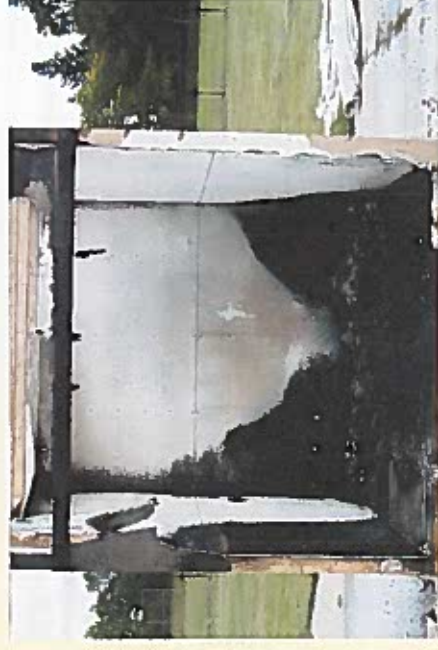
FIGURE 8-18 Postfire view after 4 minutes of gasoline-accelerated fire. The ceiling and front drywall collapsed from firefighting action. Note protected areas on walls behind both large chairs. Photo courtesy of Special Agent Mike Marquardt, CF, ATF, Grand Rapids, MI. Test courtesy of the Iowa Chapter of the IAAI.
